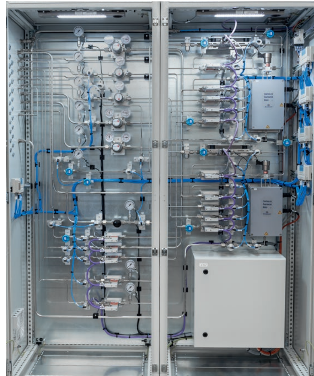
CVD Silan -Chlorine Gas Distribution – orbital welded
